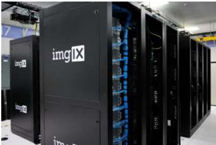
Gambar 13.10. Ruang Data Centre Sumber : imgix di https://unsplash.com/
