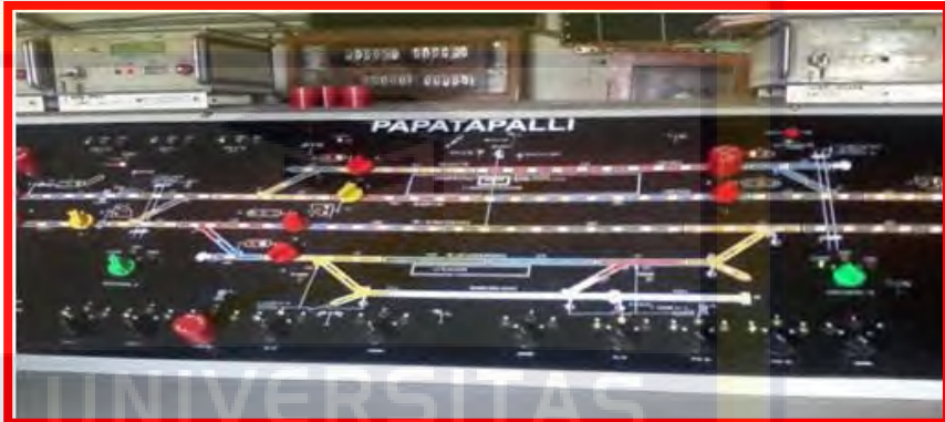
Gambar 6. 17 Local Control Panel
