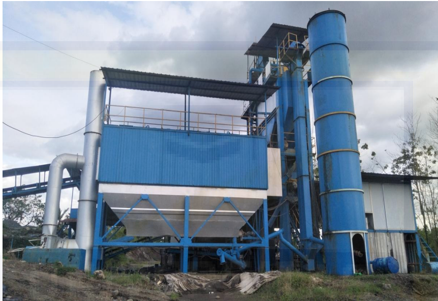
ASPHALT MIXING PLANT
