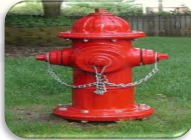
Gambar : 3.13 Water Hydrant Sumber: Google 2019
