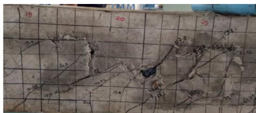
Figure 7: Spallings on the beam body
