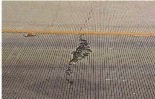
Gambar 2.23 Kerusakan gompal (Sumber : Wahid Ahmad, 2009 )
